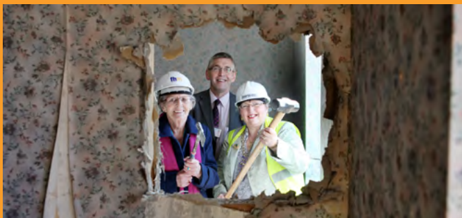
2012: Work begins - with help from some residents - as we start developing our Castle Court sheltered accommodation
